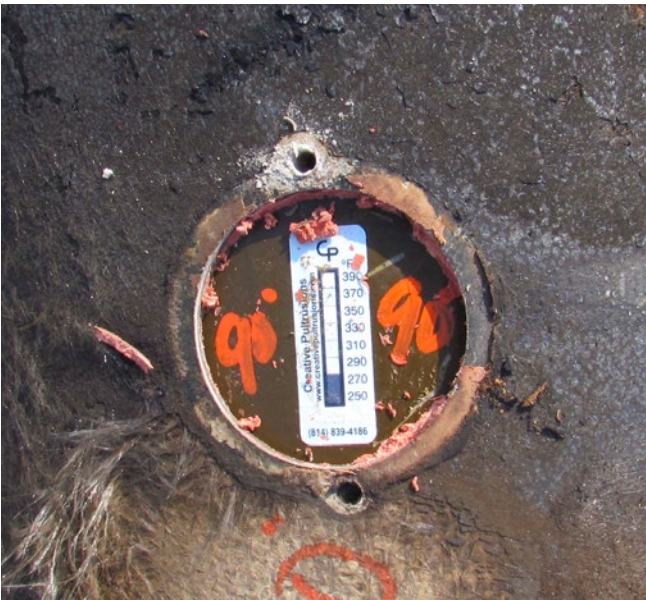
Irreversible Temperature Measuring Device after fire exposure, viewed through the fire protection sleeve.
